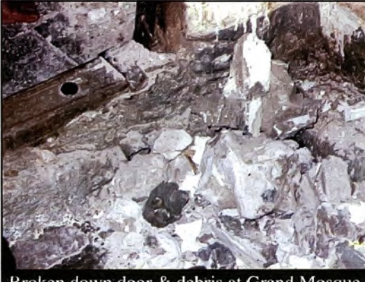
Broken down door & debris at Grand Mosque
