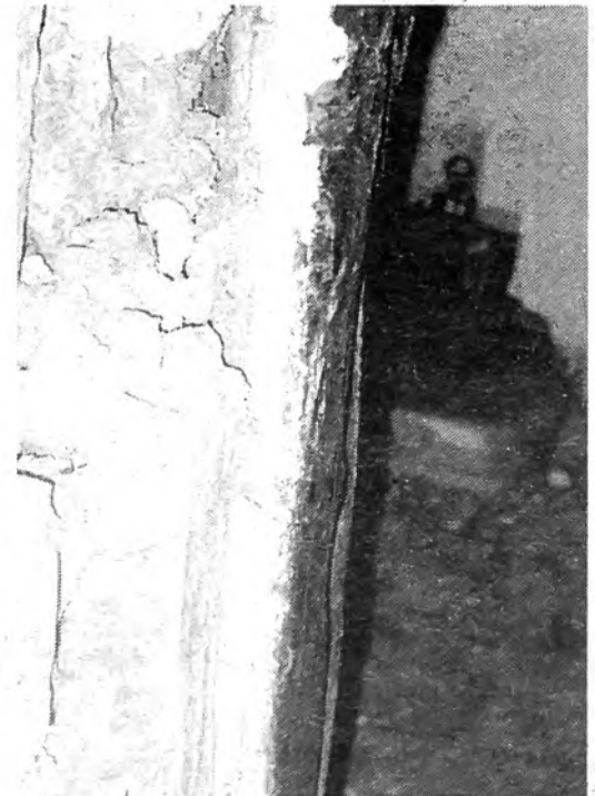
The remains of the broken door of the mosque
