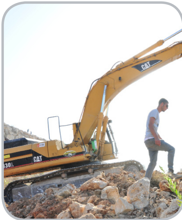
ARIEL (ISRAEL), Sept. 27 -- Construction vehicle works as the building of a housing project resumes in the West Bank Jewish settlement of Ariel. The moratorium on Israeli construction in West Bank settlements, declared by Prime Minister Benjamin Netanyahu last November, expired at midnight on Sunday. (Xinhua/Yin Dongxun)
