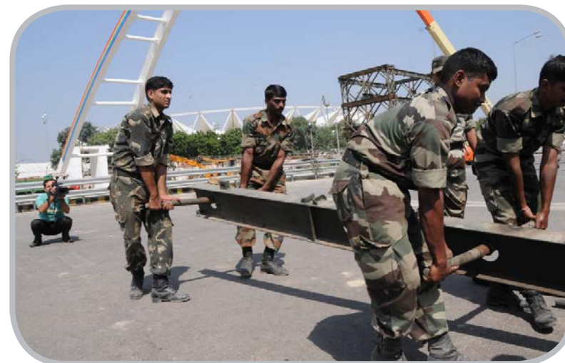
NEW DELHI, Sept. 26 -- Army personnel reconstruct the collapsed foot bridge, in New Delhi, India. The Delhi government has asked the Indian Army to build a foot bridge outside the main flagship Jawaharlal Nehru Stadium to replace the one that collapsed last Tuesday, said officials on Saturday. (Xinhua/Partha Sarkar)
