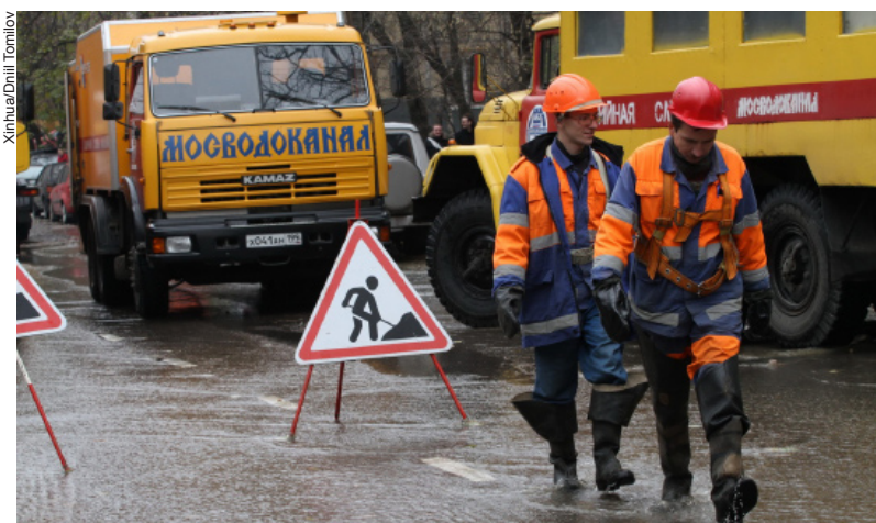
Russian rescue workers walk in water leaking from a broken pipeline at Malomoskovskaya in northeast Moscow, Oct. 26, 2010. The street was flooded and the traffic of the area had been influenced.
