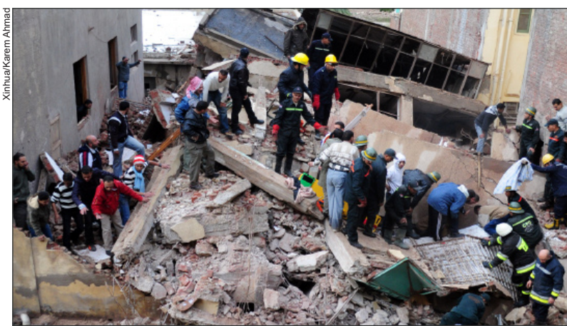
ALEXANDRIA, Dec. 12, 2010 — People search for survivors in a collapsed factory building in Alexandria, Egypt. At least three people were killed when a factory collapsed due to bad weather in Alexandria, officials said.
