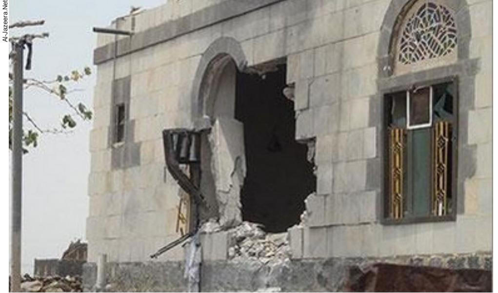
Signs of the damages in Arhab north of the capital city Sana'a where armed conflict has been going off and on for the last three months.
