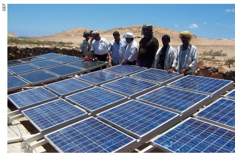
Use of Solar energy for domestic water supply in Shueb, Qalancia, Socotra funded by the GEF small grants program in 2006. The project aimed at providing community with solar pump to elevate the water 70 m to a hilltop 600 m away from source to reach the village by gravity.
