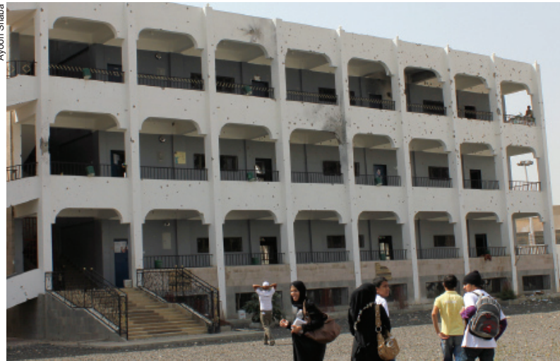
Young activists renovating Al-Rammah School in Al-Hasaba conflict zone Sana'a after it was used as by the army as a temporary military stronghold. There are other schools used by either conflicting sides depriving by that the students of their education.
