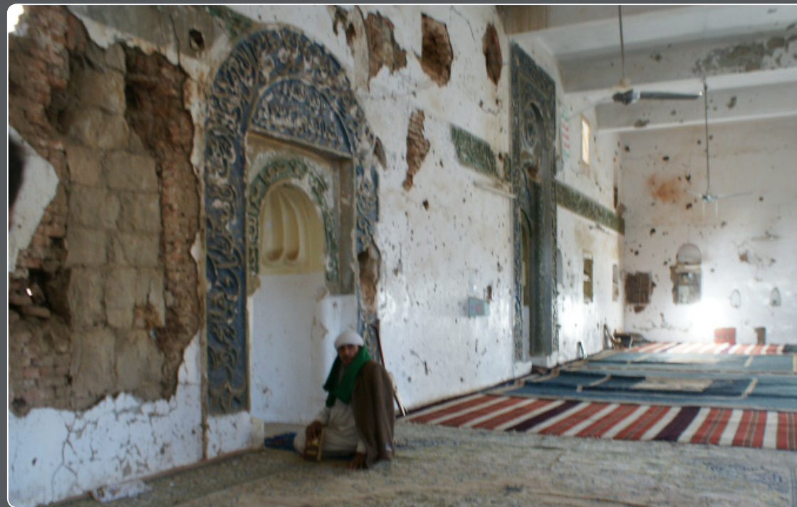
A damaged mosque at the old city in Sa'ada which was affected by the shelling between government and Houthi armed groups in 2008.
