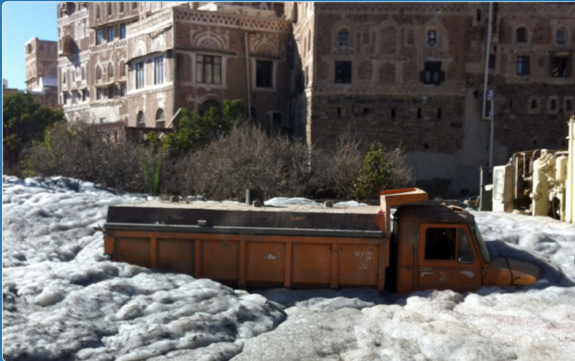
Drilling for a new well in the Old City goes wrong, stranding workmen and trucks in a sea of bubbles. Photo by Garnet Roach
