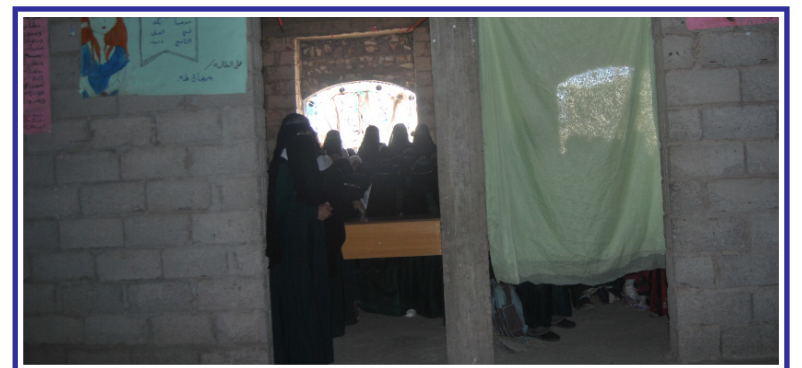
The school administration has resorted to using curtains in place of doors.
