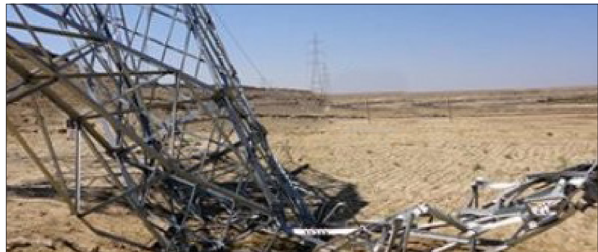
Marib has been the constant target of pipeline attacks.
