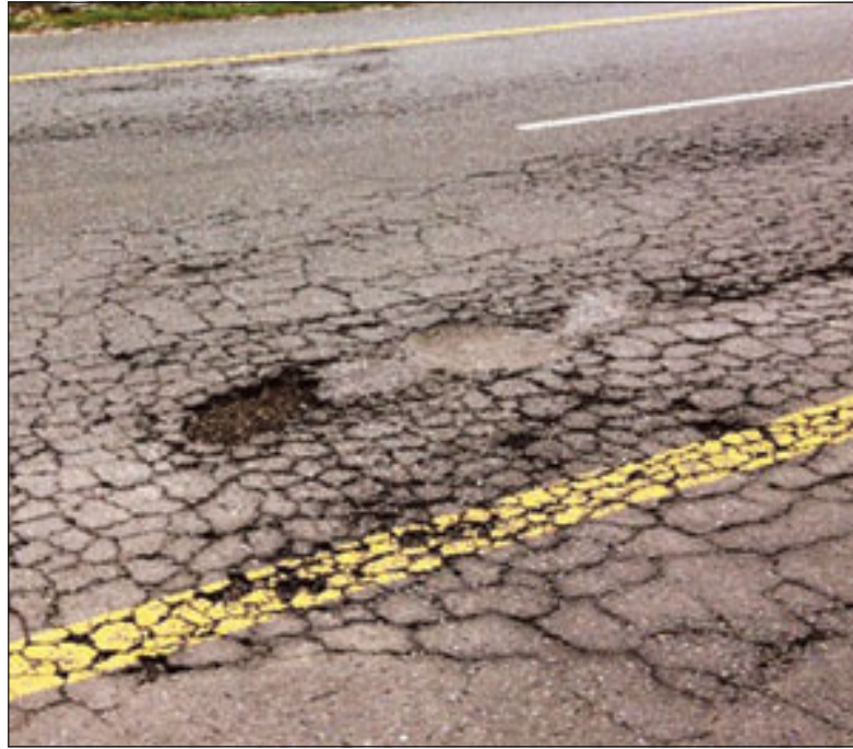
Holes like this are typical on roads across Sana'a.
