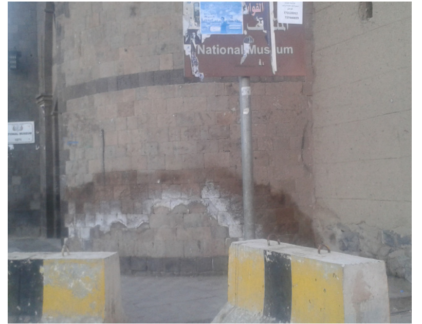
A national museum wall frequently used as a "toilet" is now in a state of decay.
