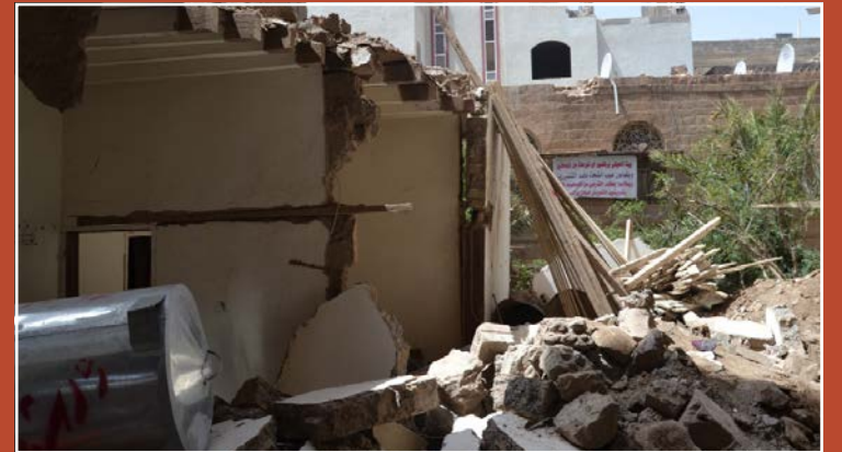
Some residents say they have no idea how long rebuilding efforts will take.
