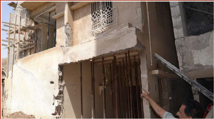
Houses were devastated by the crash. Mohammad Al-Yamani points at the crumbling exterior of a neighborhood house.
