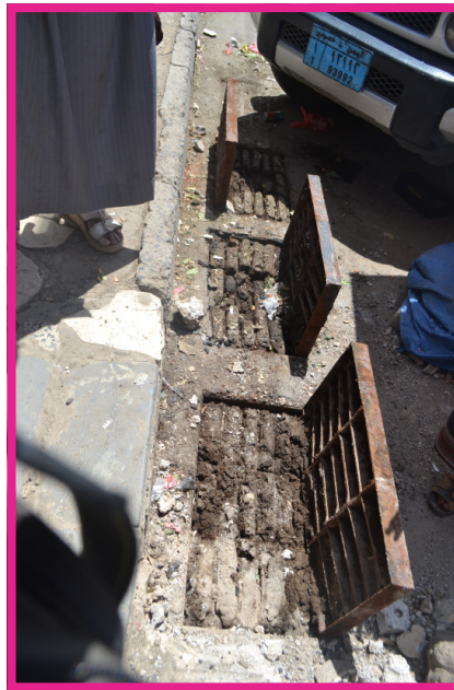
Rain traps filled with dirt and debris are found all over Sana'a.
