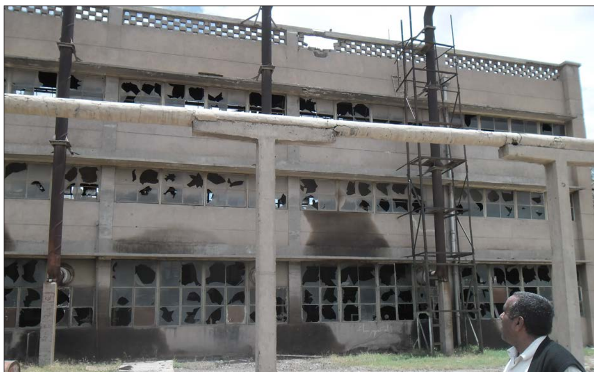
The factory used to provide housing for its workers. It's the same building that housed the original construction crew that built the factory in 1964. No renovations have ever been made on the building.
