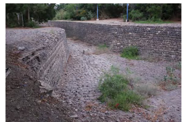
Local authorities in Aden are working on a renovation plan for the cisterns, some of which have fallen into disrepair.
