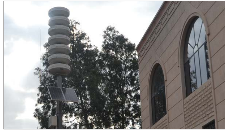
USAID paid for the solar equipment at the Bilquis Club. Now the sporting facility is in charge of maintaining it.
