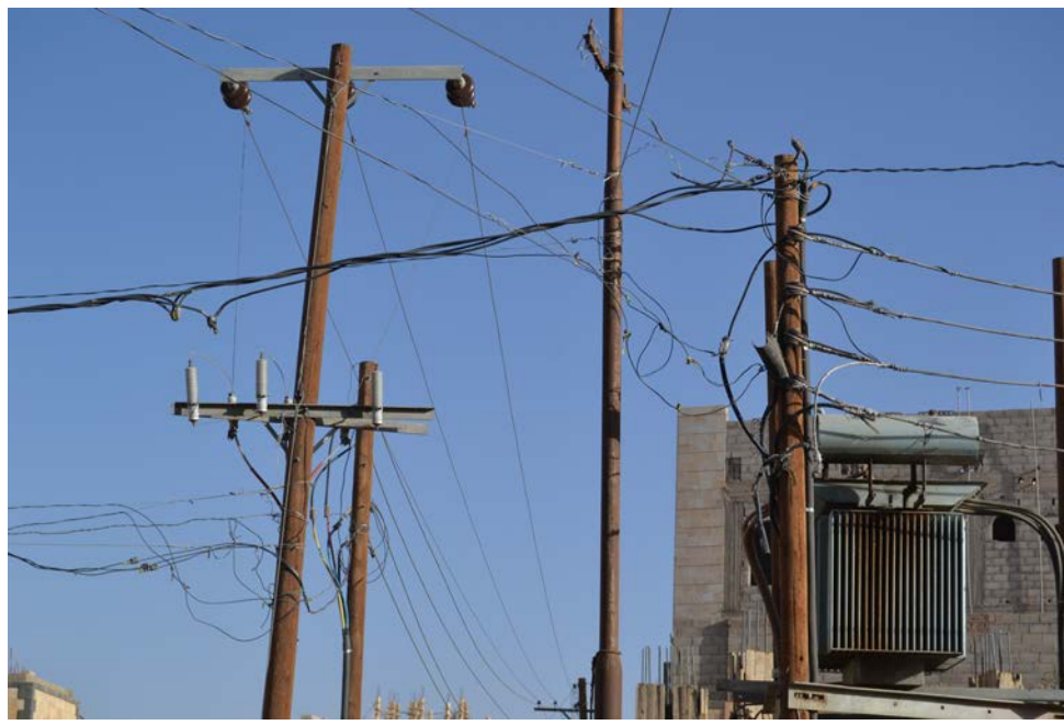
Illegal tapping into electricity lines comes at a great risk: Every day cases of injuries or deaths caused by electrical shocks are registered at Sana'ani hospitals.
