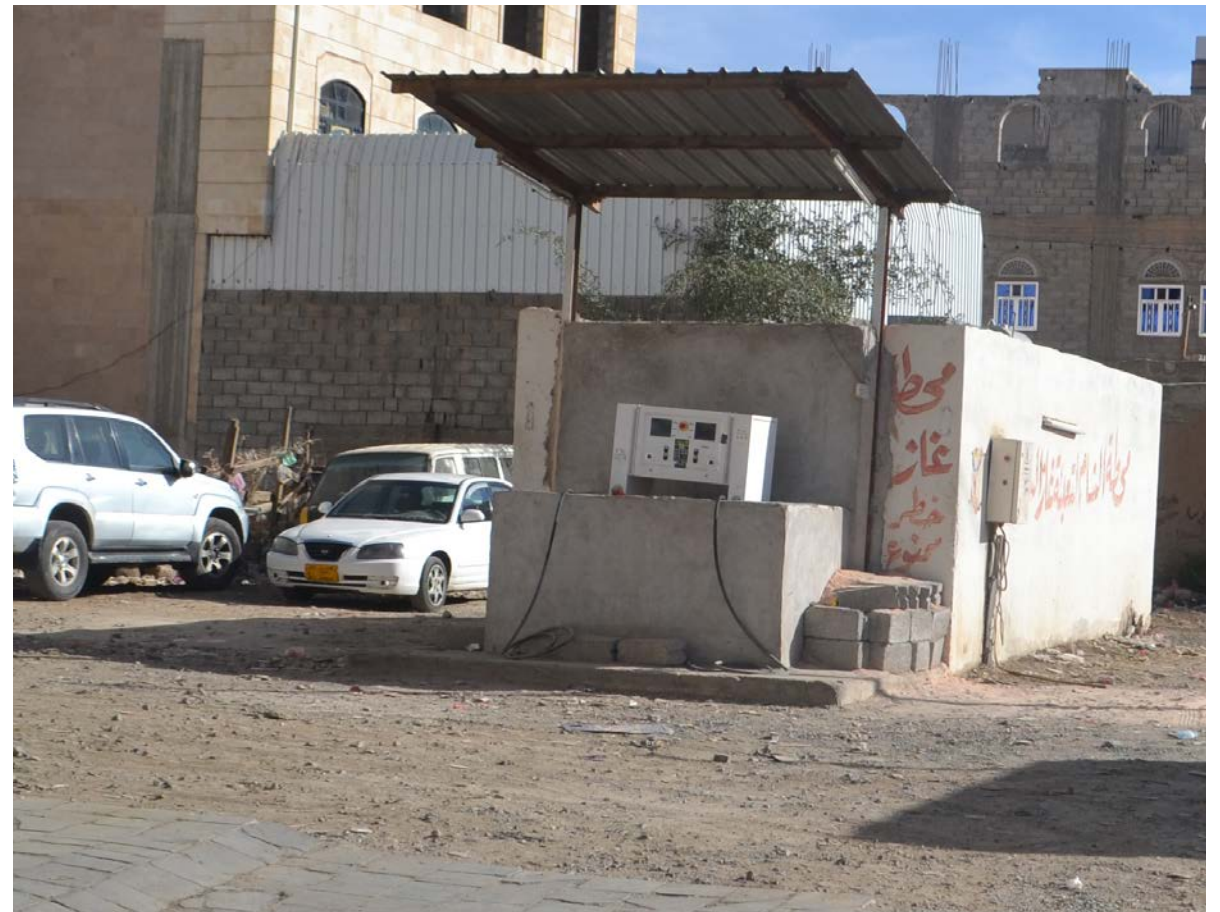
Since 2011, the number of unlicensed gas stations in the capital has boomed. Officials say they are preoccupied with more pressing concerns, but residents fear for their safety. Clashes, car bombs and other explosions leave Sana'a in even greater danger of lethal accidents, some have pointed out.
