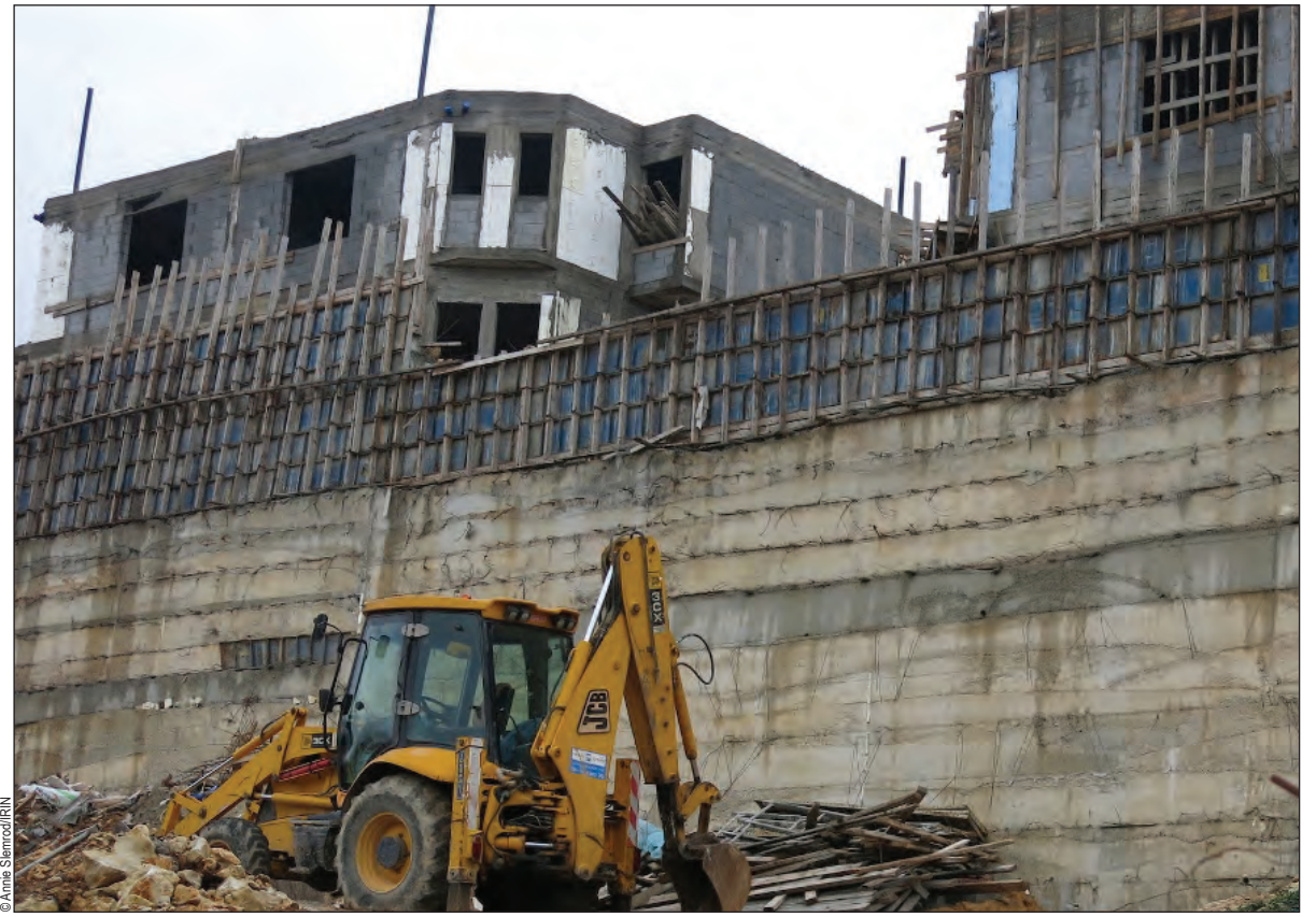
Construction workers in the West Bank settlement of Ariel. Declared illegal by the UN, such Israeli settlements have expanded in recent years.
