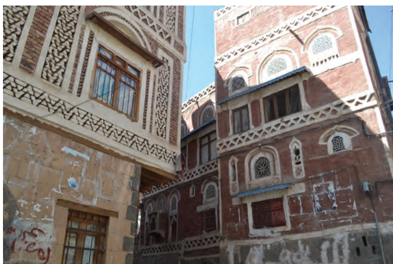
The bricks used to construct the first story on each of these buildings violate the traditional Old City style architecture.
