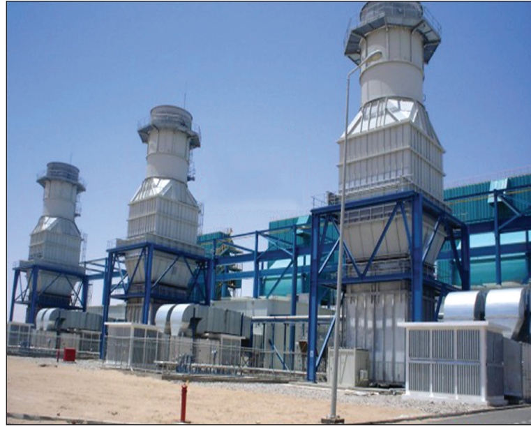
The gas-operated plant in Marib governorate supplies approximately 40 percent of Yemen's energy needs. Experts estimate it will be out of use within 16,000 hours at most unless urgent repairs are made.
