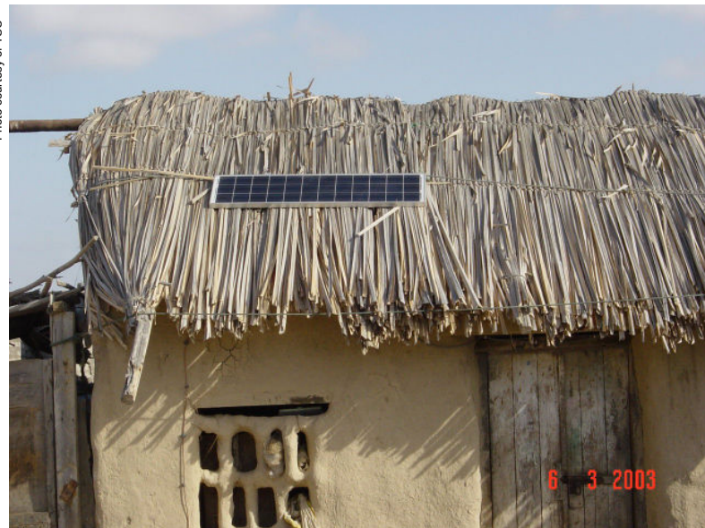
Most of TSC's renewable energy systems are installed in rural areas where there is no electricity.
