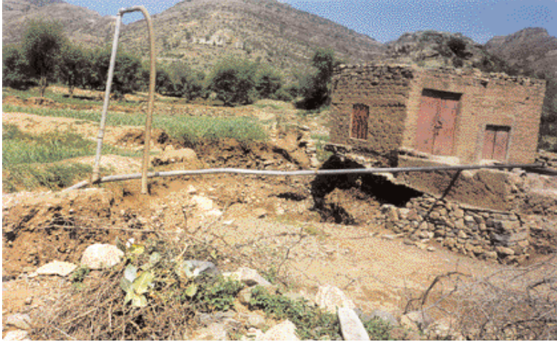
A brick house became unsafe after the heavy rain
