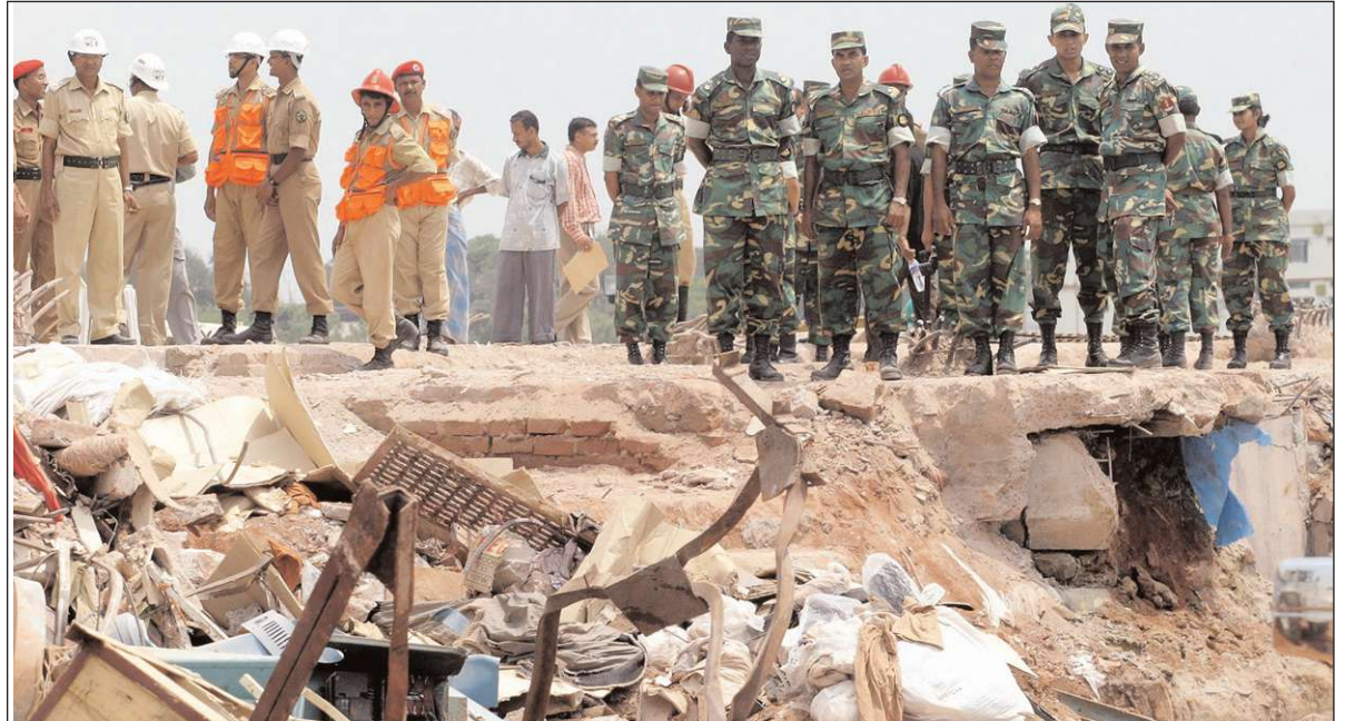
Soldiers and other rescue workers stand at the site of the collapsed nine-storey garment factory after ending the search for victims near Dhaka April 19. REUTERS
