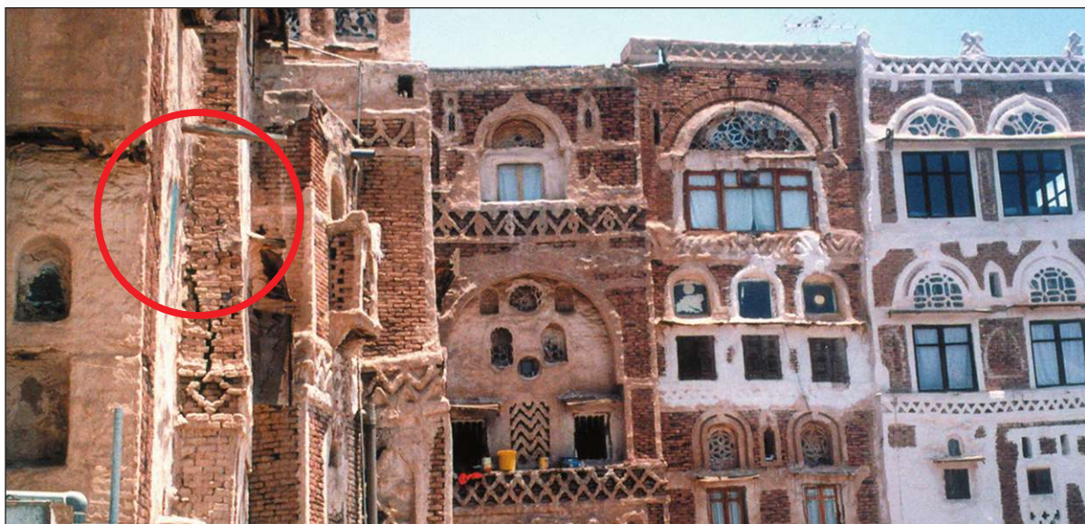
Cracks crawl on the walls of the old city, threatening an imminent collapse
