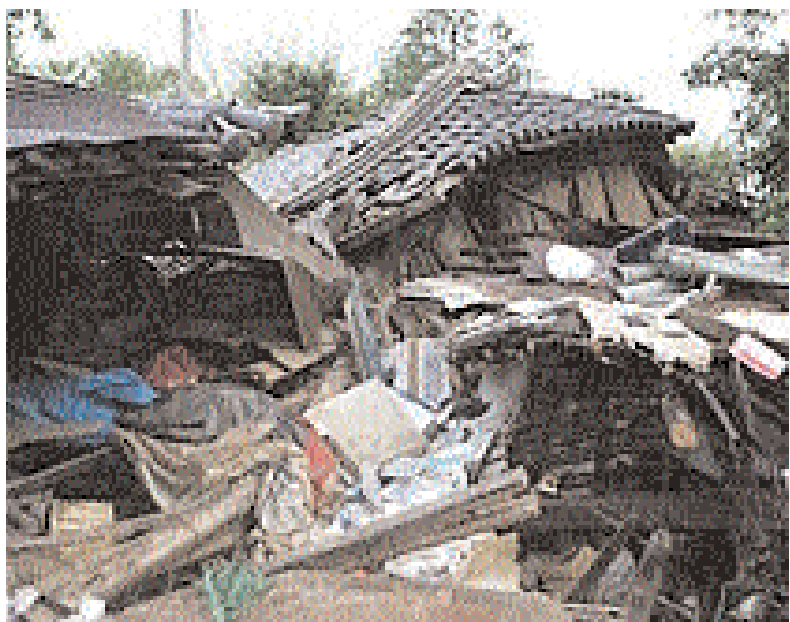
A collapsed house lies on the ground following a quake that shook earlier Tuesday, Aug. 16.
