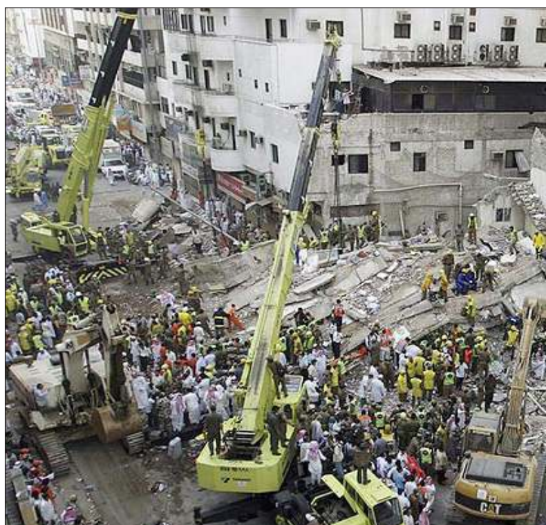
Rubbles of the collapsed hotel in Mecca.
