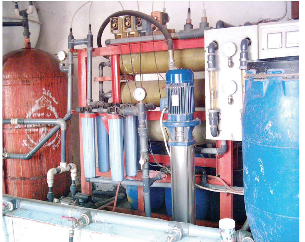
Equipments in bad state in one of the purification station in Hodeidah.
