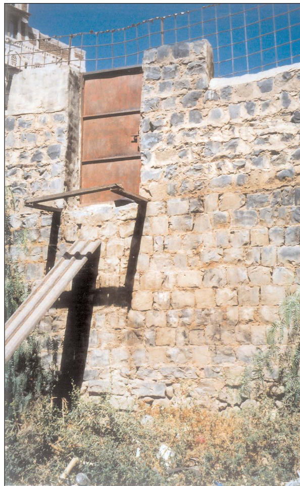
The church from inside: Shrubs have grown at the drain-wet bottom and the iron plate used by children to slip into the pit can be seen
