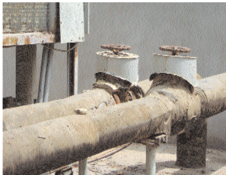
Pipes in the central ventilator are subject to constant breakdowns and the biggest problem is that most spare parts are unavailable.
