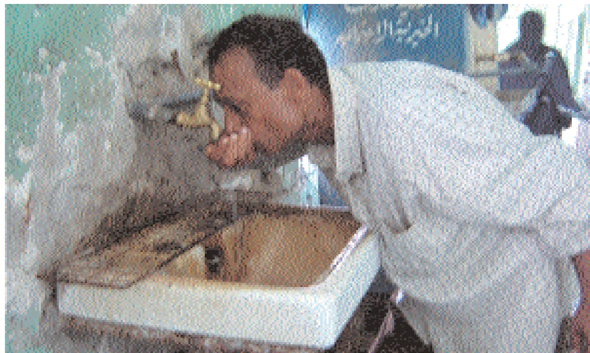
A nurse drinks directly from the tap of a rusty basin. The hospital also experiences constant water cuts.
