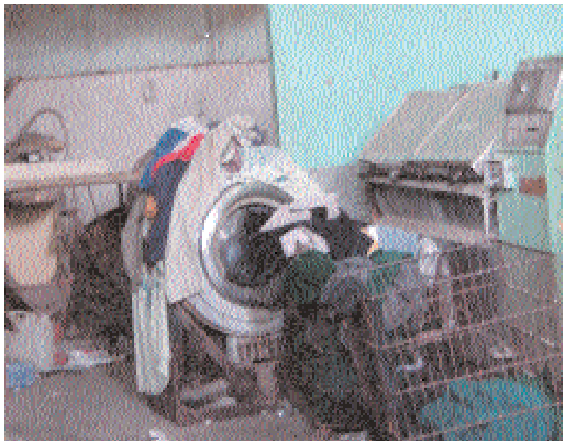
One laundry machine works in the laundry department, where blankets and clothes of medical staff and patients at the hospital are washed with only hot water and one type of soap.
