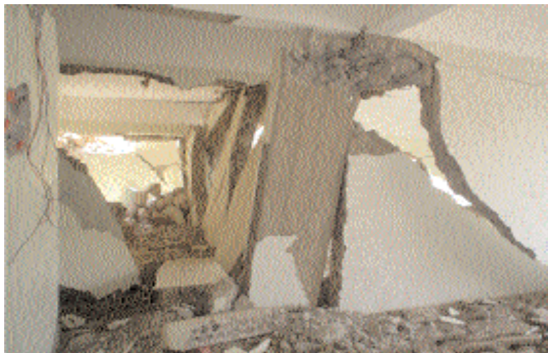
The resulting damage of a collapsed house in Taiz.
