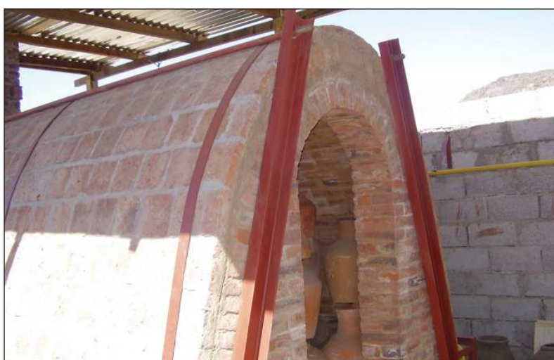
The kiln will not just produce clay pots, but also irrigation ceramics and water filters.
