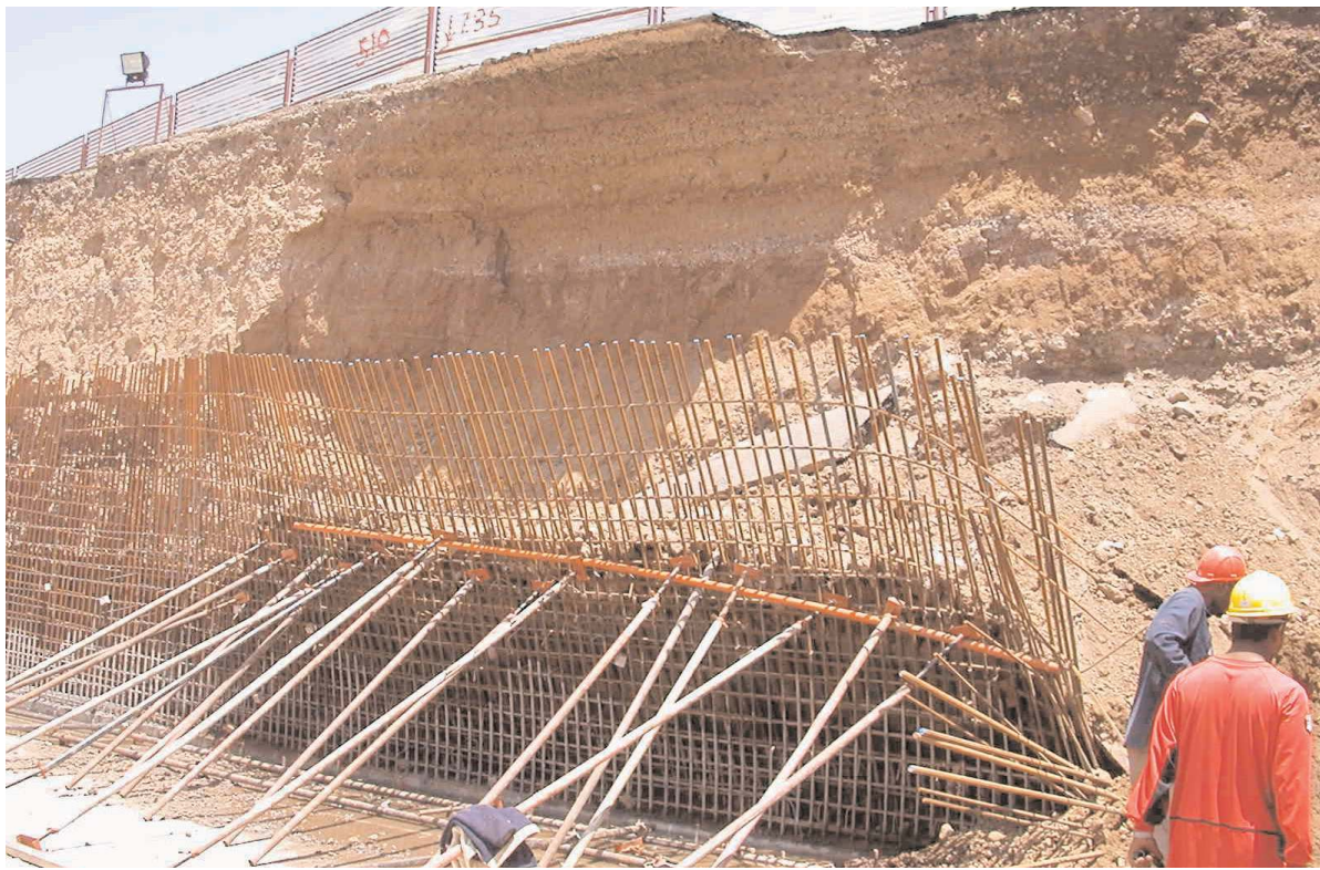
Iron bars have been used in order to support the structure bent because of the collapsing muds.
