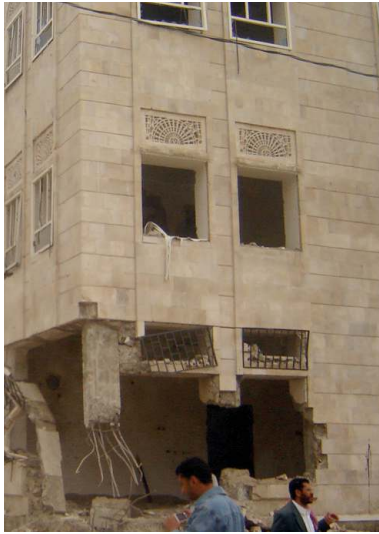
Almost all government buildings and houses are damaged in Sa'ada.
