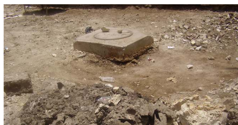
The drain issue, in the Old City of Sana’a, is a disaster. “Before a day, water filled this place,” Hassan Lutf, director of the local council in the Old City, stated.
