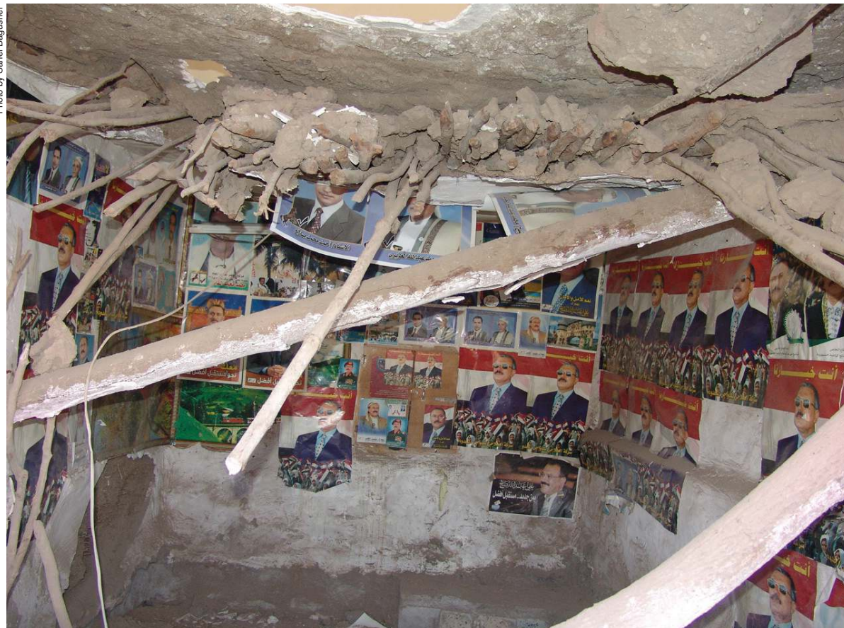
This room, plastered with posters of President Ali Abdullah Salih, collapsed in December, displacing a family of 19.
