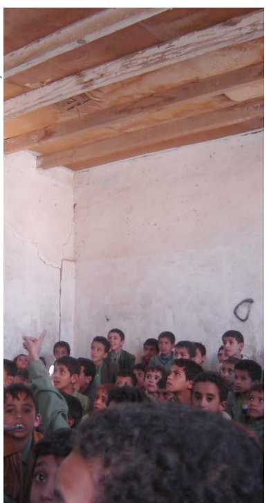
This classroom used to be a bathroom. Its roof is likely to collapse.
