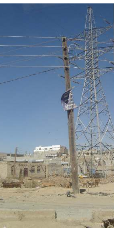
Unstable power lines can be seen in the middle of the neighborhood.
