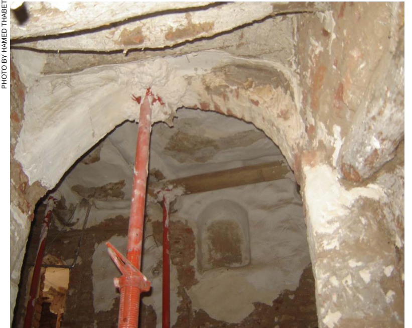
Many residents are afraid to return to their homes because of the danger of collapse during the rainy season. Some of them returned to their destroyed houses, because they have no other choices.
