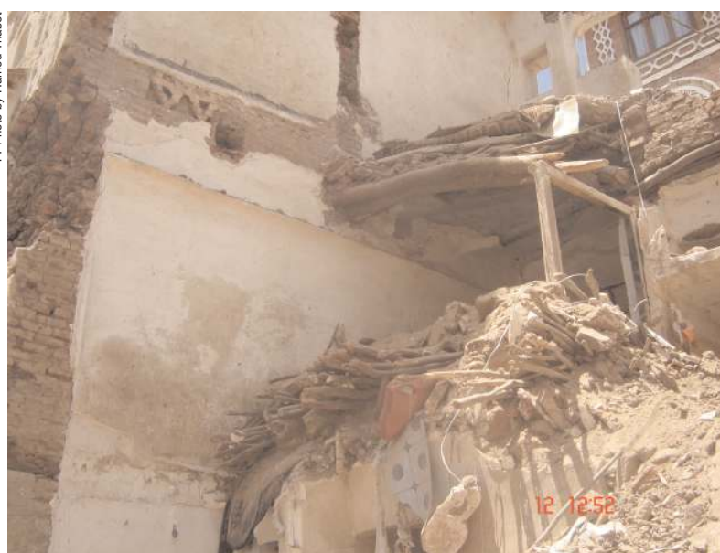
The collapse causes two deaths in the old city of Sana'a.
