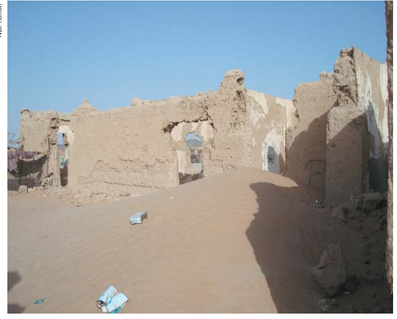
Beer Al-Marazeeq School in Al-Jawf built in 1989, has been made to ruins because of conflict and exchange of firearms. Now the school instead of hosting its students is a shed for goats.
