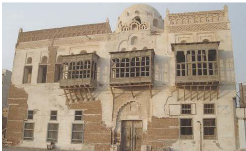
Nothing remains in the museum except for rust that tells the terrible story of the ancient building that has become dilapidated because of neglect.
