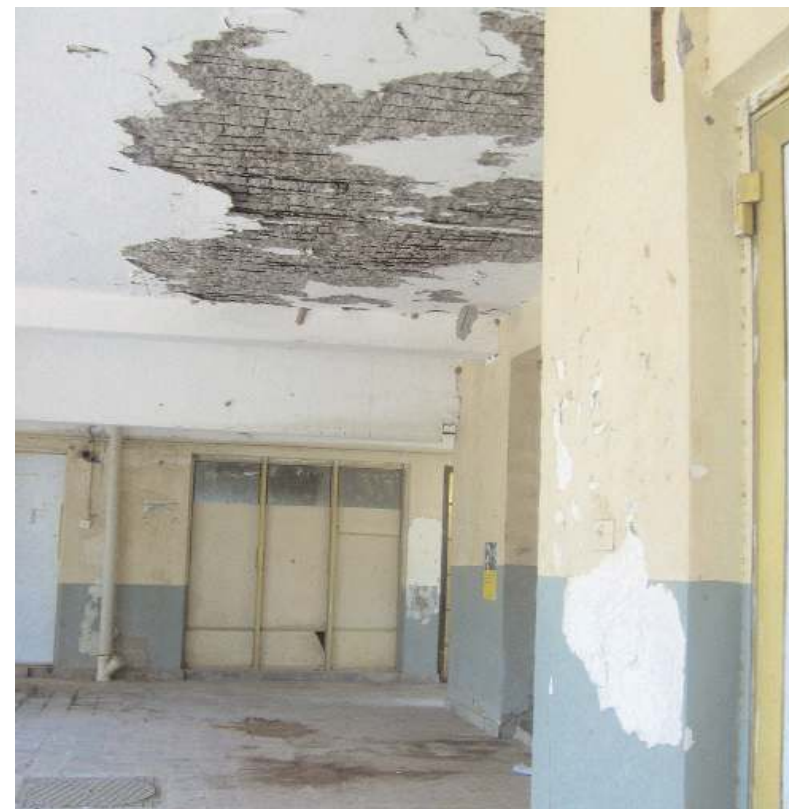
The media department, which is part of the Faculty of Arts, is located in an unstable facility full of breaches and clefts.
