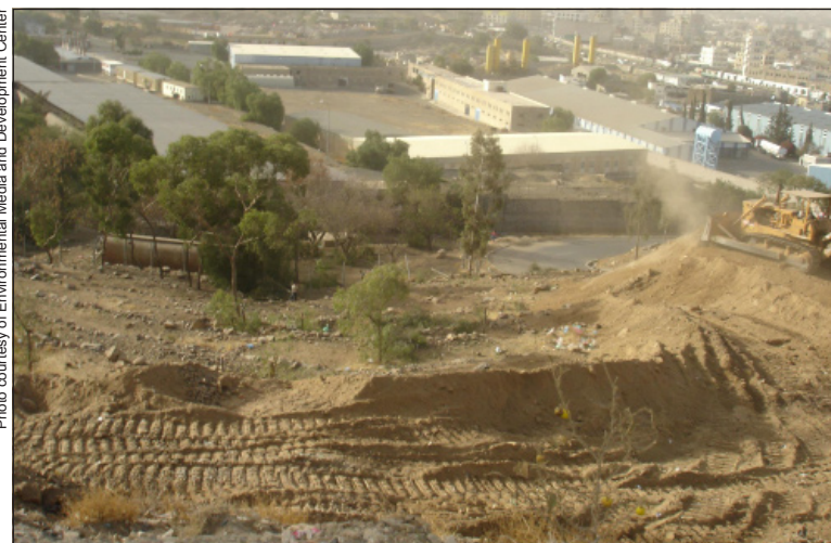
Bulldozers of the capital secretariat damage trees in Faj Atan district in Sana'a The source of the picture is Environmental Media and Development Center
