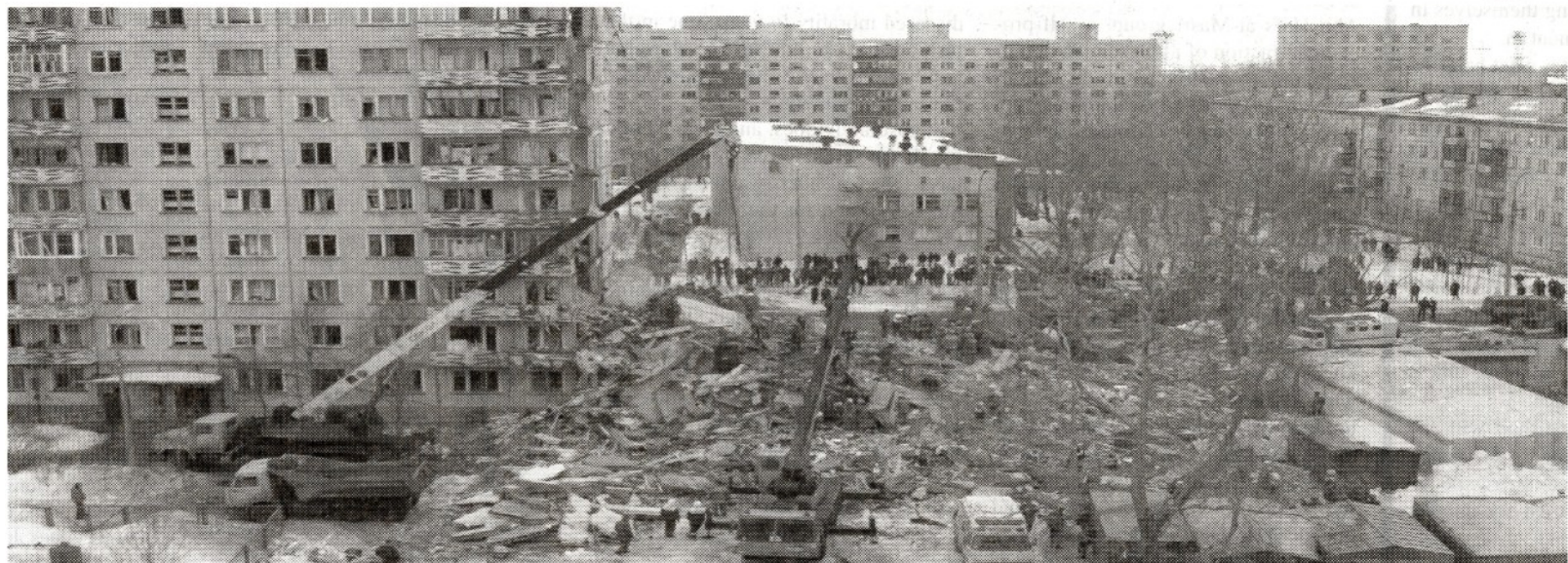
General view of the blast site in Arkhangelsk, Mar. 16. A night-time explosion, almost certainly caused by a gas leak, levelled part of a large apartment block in northern Russian on Tuesday, killing at least four people with 70 missing beneath rubble, officials said. REUTERS
