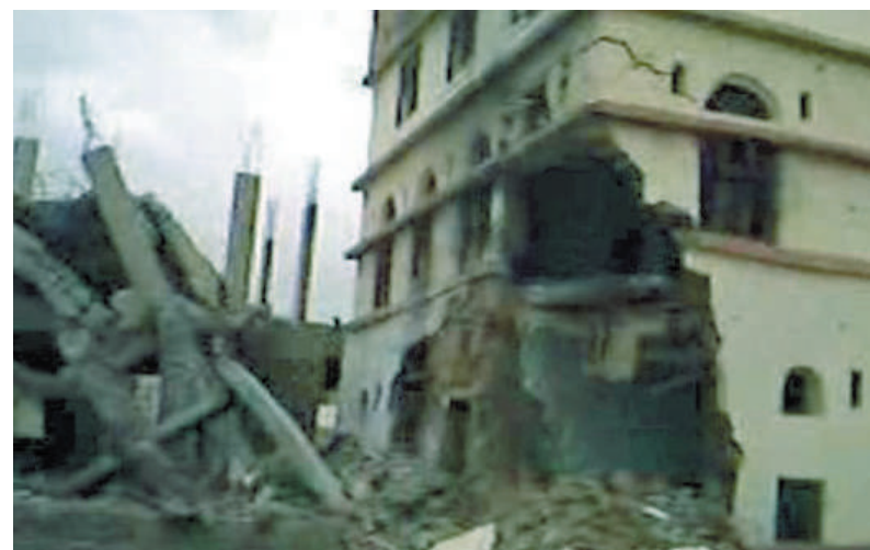
An official report revealed that the Sa'ada war left more than 4,000 homes damaged and more than 200 public facilities partially or completely destroyed.
