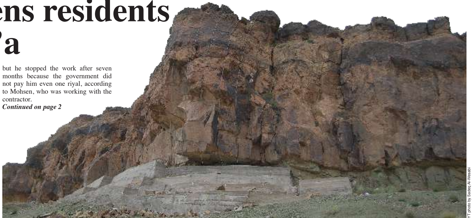
A large outcropping of rock in Sana village just half an hour from the capital's city center, has been threatening a village of around 1,000 inhabitants.
