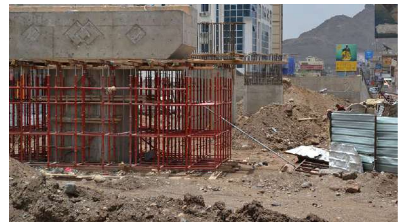
Many bridge columns have yet to be constructed. Workers digging holes for the columns struck a water tank, creating delays in the construction process.
