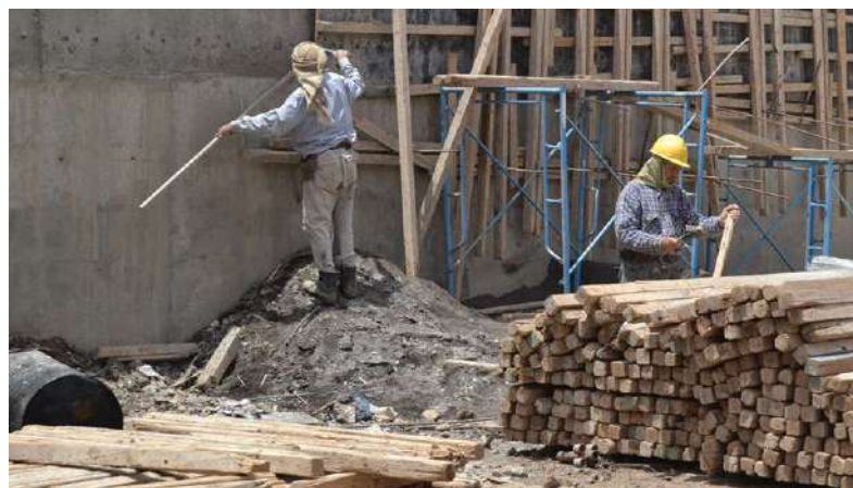
Carpenters Ali and Mohammed working on the entrance of the tunnel. They have been working in this field for over 25 years.
