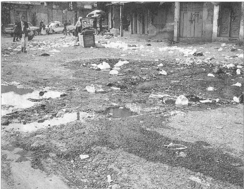
Some streets in need of repair
