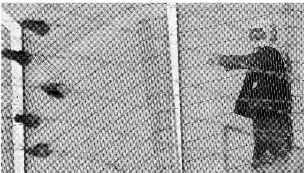
Palestinian man walks by an electrified security fence that is under construction by the Israeli army to separate Bethlehem from Jerusalem July 29, 2003. Israeli Prime Minister Ariel Sharon will try in talks with U.S. President George W. Bush on Tuesday to ease his concerns about a planned West Bank security fence that Palestinians condemn as a land grab. REUTERS
