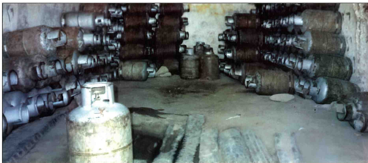
Gas shops, lack of safety procedures
